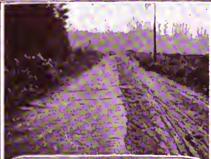
Over Decadent Planks— Divers Planks Missing.
